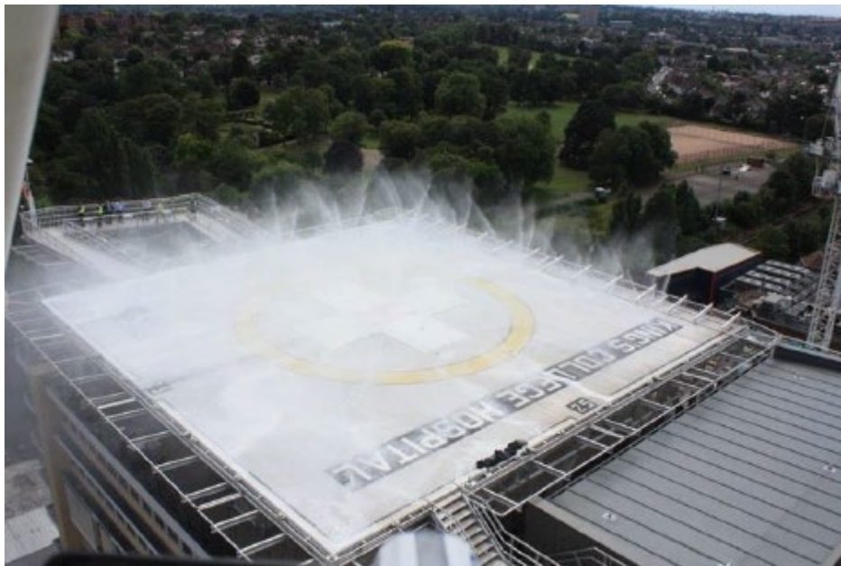
Figure II-6-5. A foam DIFFS on a solid plate surface at an elevated heliport
