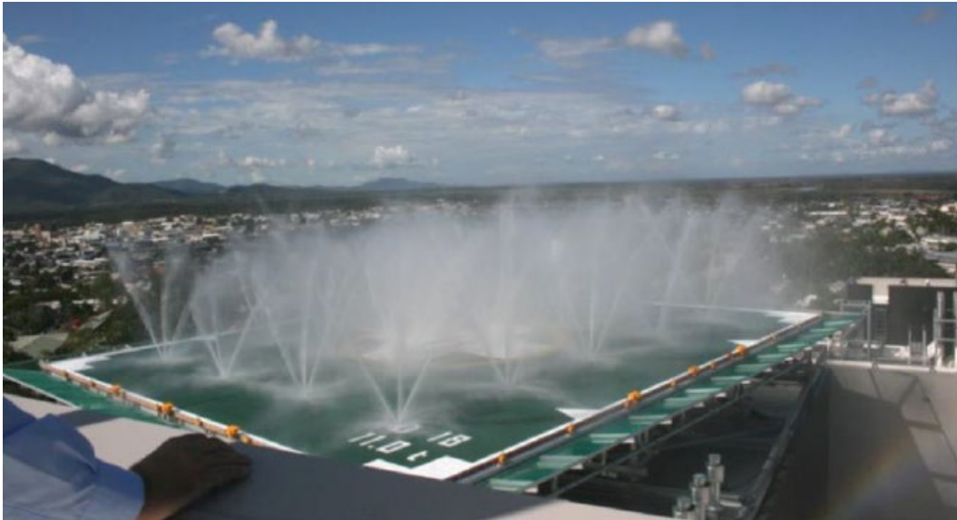
Figure II-6-8. A water-only DIFFS on a heliport with a passive fire-retarding surface
