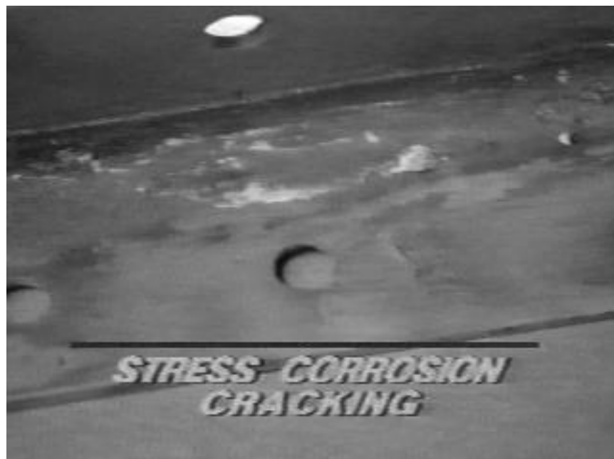
Figure III-9-74. Stress corrosion cracking may be identified by the presence of multiple, fine cracks in high-strength alloys.
