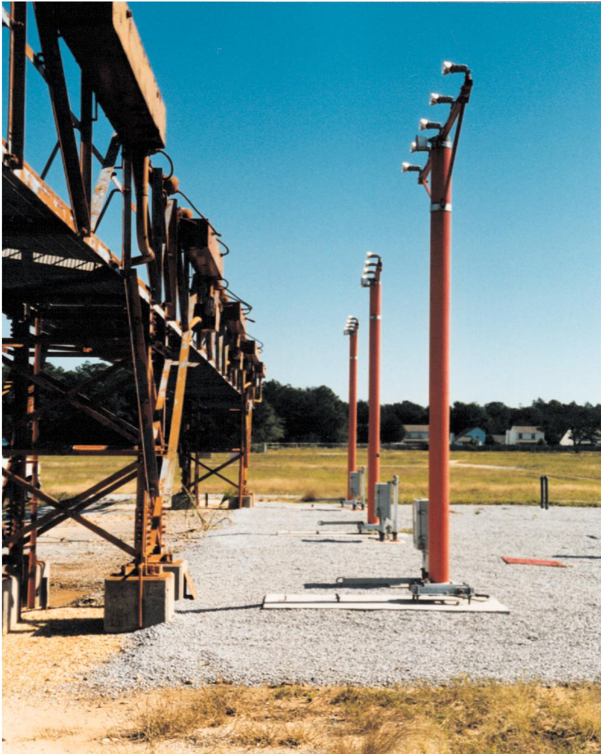
Figure 4-6. Approach lighting station of rigid design (left) being replaced by new frangible structures (right)
