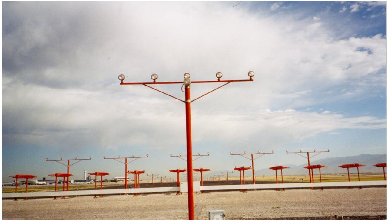
Figure 4-3. Approach lighting towers — fibreglass tubular poles
