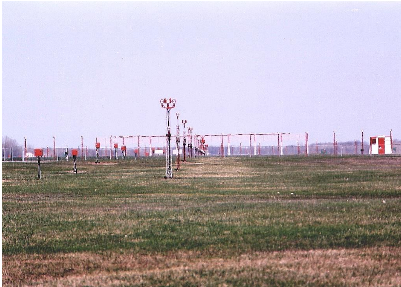
Figure 4-4. Approach lighting towers — aluminium lattice structures
