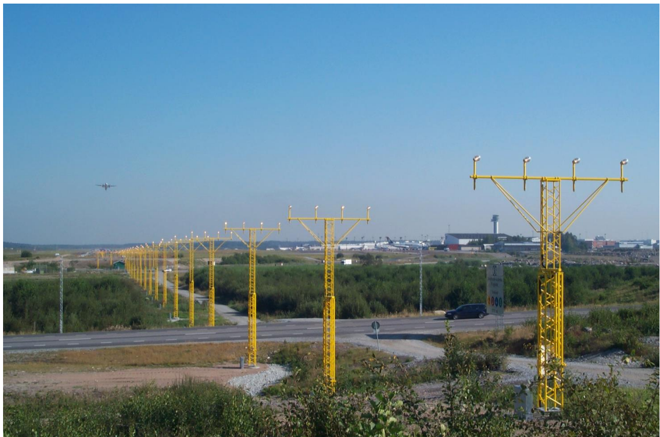
Figure 4-2. Approach lighting towers — fibreglass lattice structures
