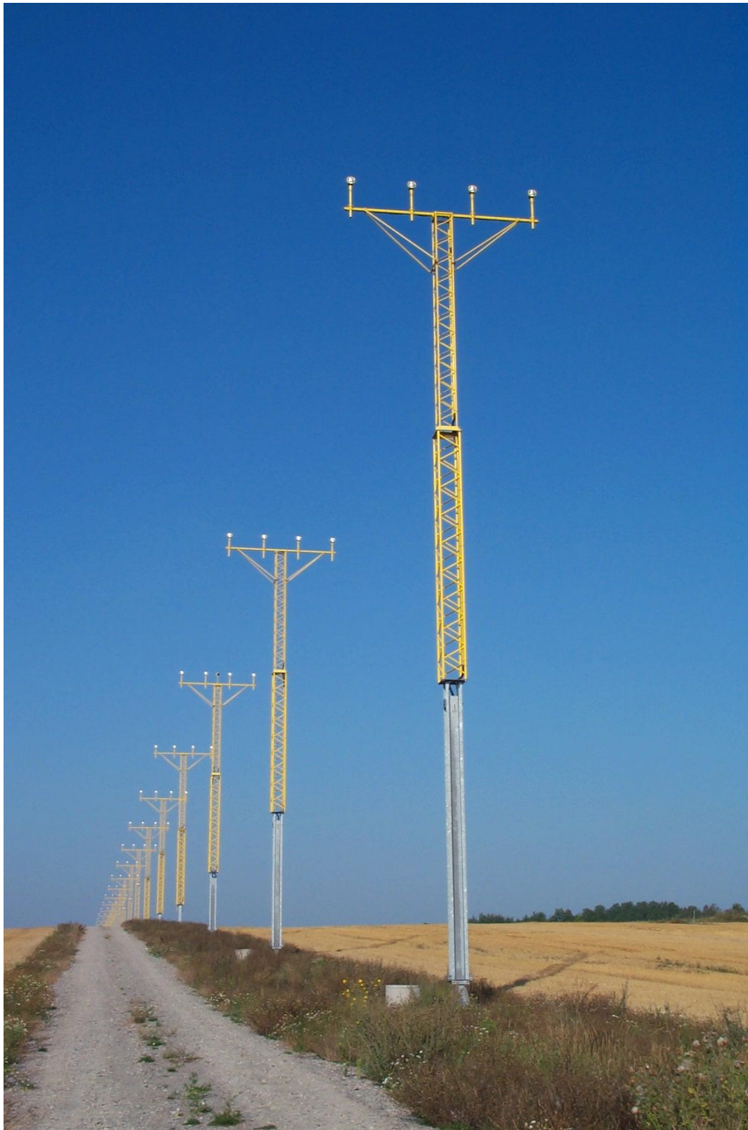
Figure 4-8. Fibreglass approach lighting towers on rigid supporting structures
