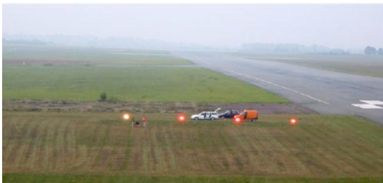
Figure 8-16. PAPI as seen from lift platform Photo source: STAC, France
