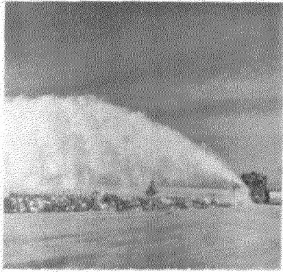
7. Snow blower clearing light windrow of snow over runway lights which are marked by green spruce trees.
