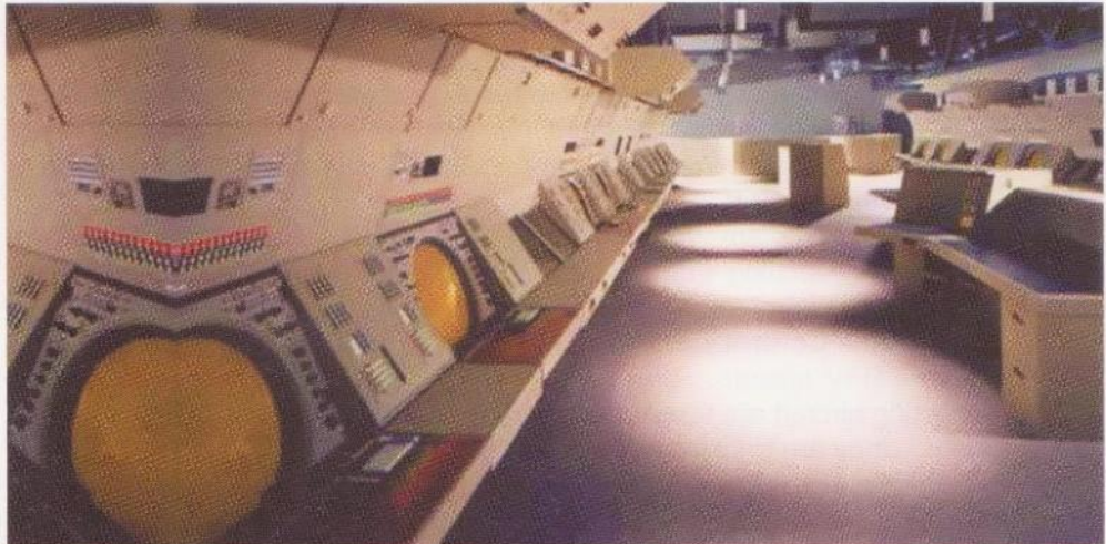
Figure 5.18 Area Control Centre.
