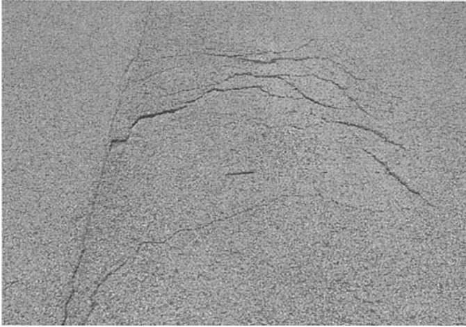
Figure D-15. Slippage Cracking.
