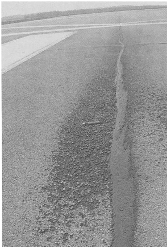
Figure D-6. Jet Blast Erosion.
