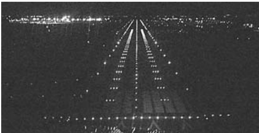
Figure 4-17. In-runway lighting at Daytona Beach International Airport. (Photo: J. Lukasik)
