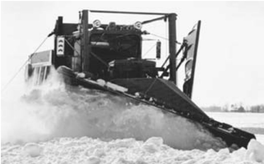
Figure 7-4. Snowplows move the snow to the pavement edges where snowblowers disperse the windrowed snow. (Photo courtesy FAA)
